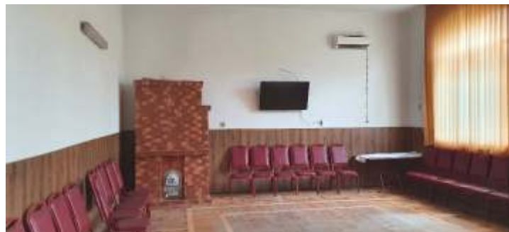
The House of Culture-City Library of the Liteni town. Stove heating system
