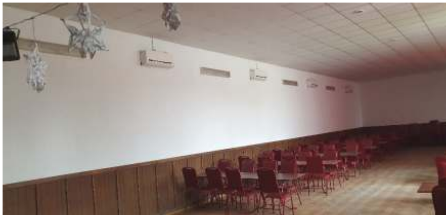
The House of Culture-City Library of the Liteni town. Inverter heating system
